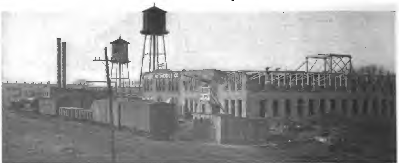
Nearly Completed Four-Story Addition to the Plant of the Moline Automobile Company, Moline, Illinois
